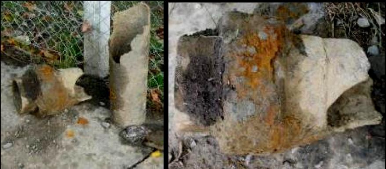
c) Fractured DN 150 (6") CI pipe
