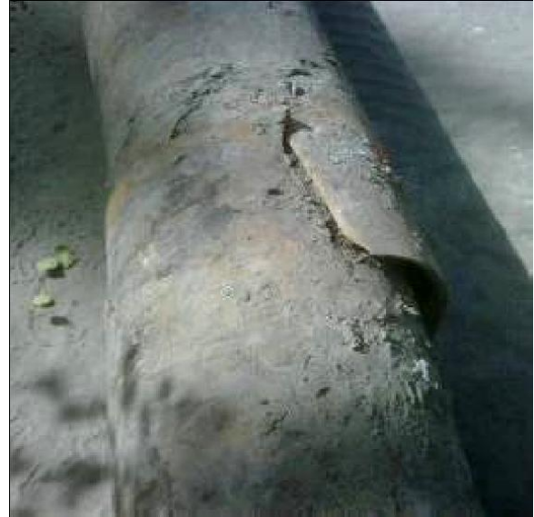
b) DN 300 (12") CLS (Concrete Lined Steel) Pipe Split (Photo by P. Free)
